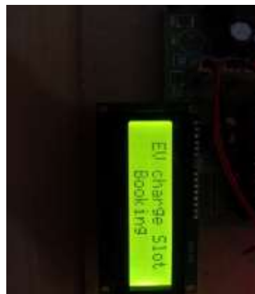
Figure.2: LCD Display the EV Charging Slot
